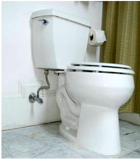
Figure 3: Flexible hose (Source: Picture by Iris D. Tommelein, Boston, MA, 2007)
