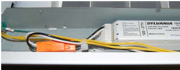
Figure 5: Wiring plug for ballast inside light fixture (Source: Picture by Iris D. Tommelein taken at Finelite, Union City, CA, 2008)
