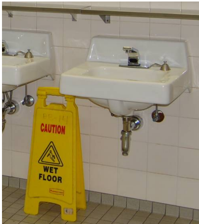
Figure 11: 'Bare' Sink in San Francisco Airport, California (© 2006 Iris D. Tommelein)
